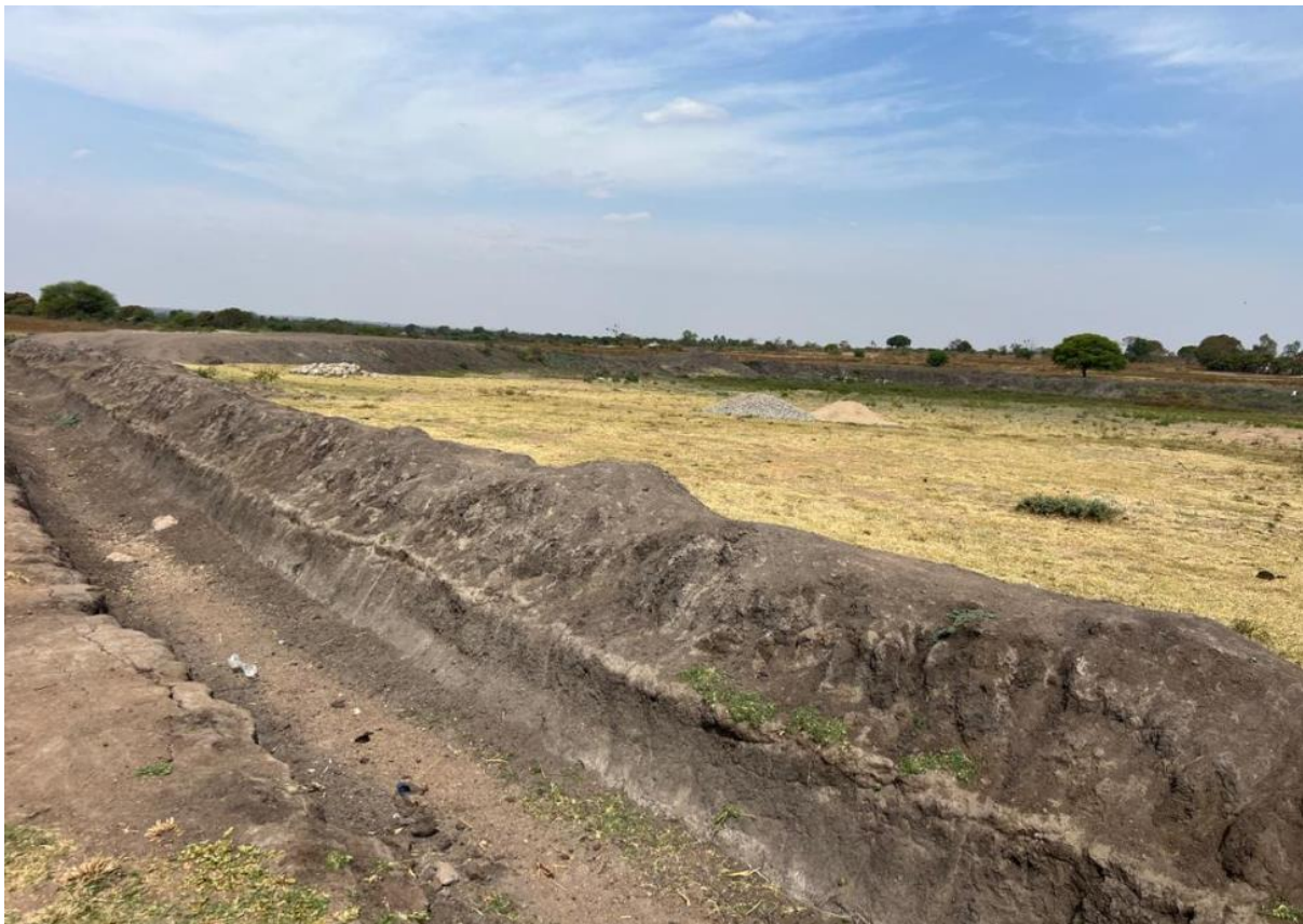
Plate 5: The rehabilitation of the charcoal dam in Nyang'anga Village would significantly improve water availability for livestock, especially during dry seasons
